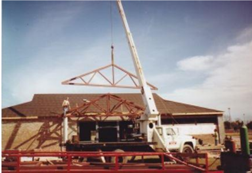
Construction on the Harrell Memorial Public Library which opened to the public in 1992.
